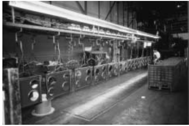
Figure 1. Present main top loading area after installation of Angle Pivoting hanging system.
